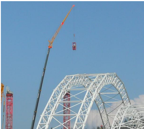
1 Exiting a work cage is a safe alternative to climbing a truss 85 m up to the framework intersection of the arch construction
